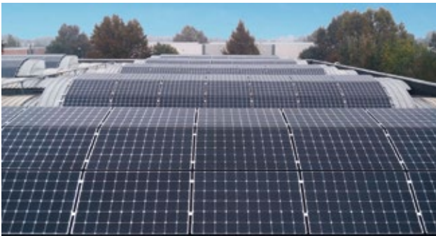
COMPACTMETAL, 80 kWp, Italy
