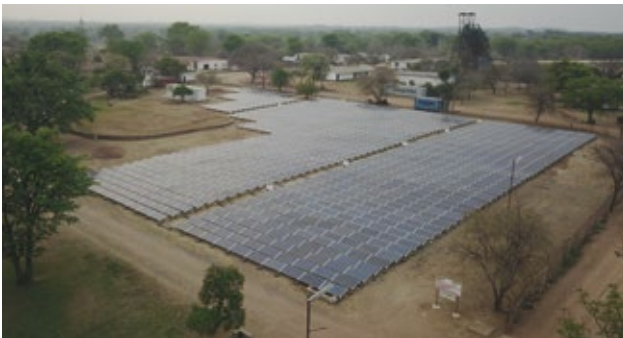
COMPACTGROUND, 500 kWp, Zimbabwe
