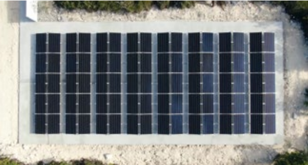
COMPACTGROUND, 32 kWp, Caribbean Islands
