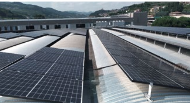
COMPACTFLAT, 120 kWp, Italy
