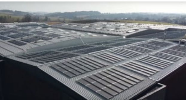
COMPACTMETAL, 1,236 kWp, Austria
